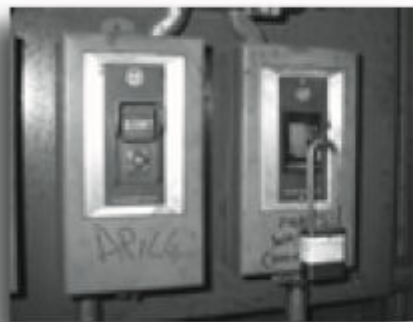
Main disconnect switch
