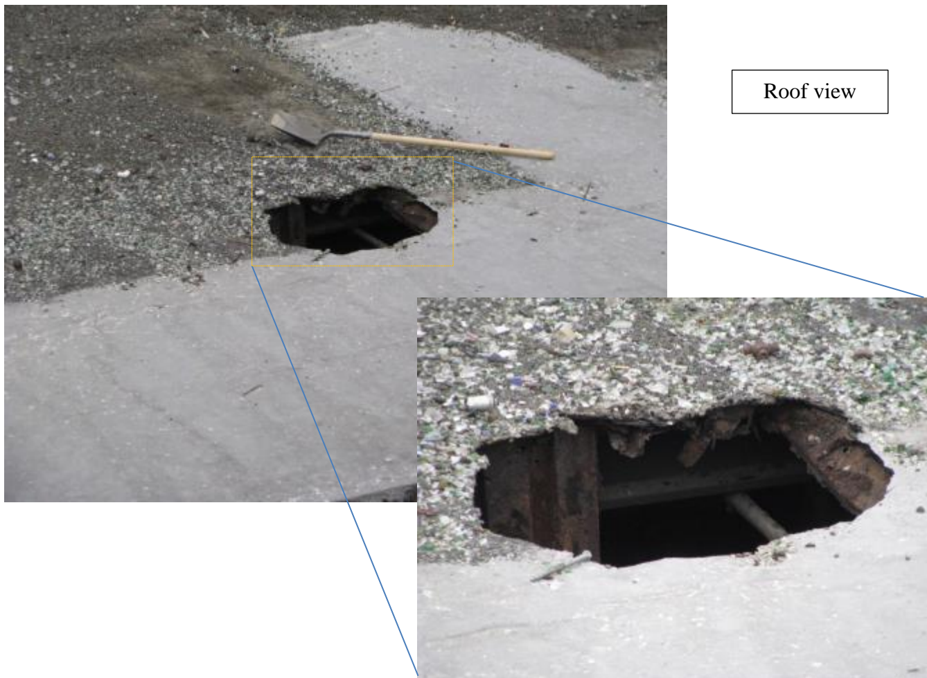
FIGURE 3. Close up of roof where victim fell.
