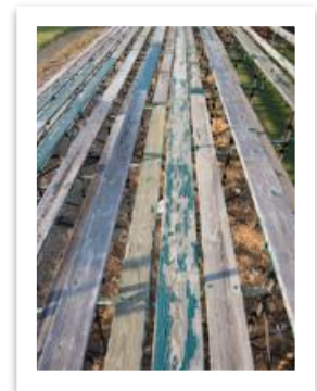
Older bleachers may become structurally unsafe.
