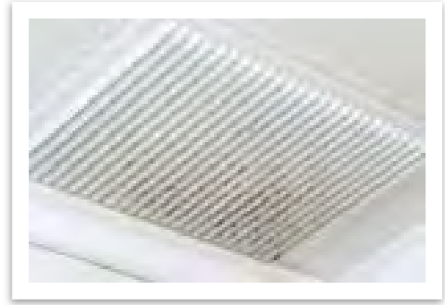
A ventilation system, such as this one, is an example of an engineering control.
