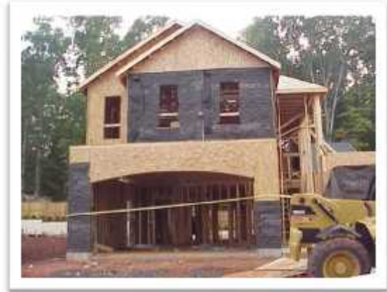
This photograph shows the two-story home workers were framing when the accident occurred.
