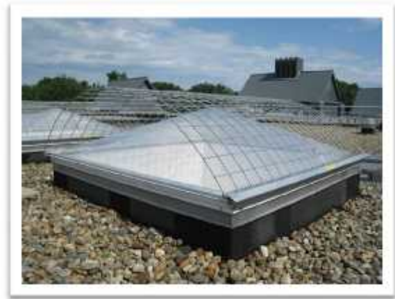
Skylight covers are necessary to protect workers. Courtesy: Simplified Safety www.simplifiedsafety.com
