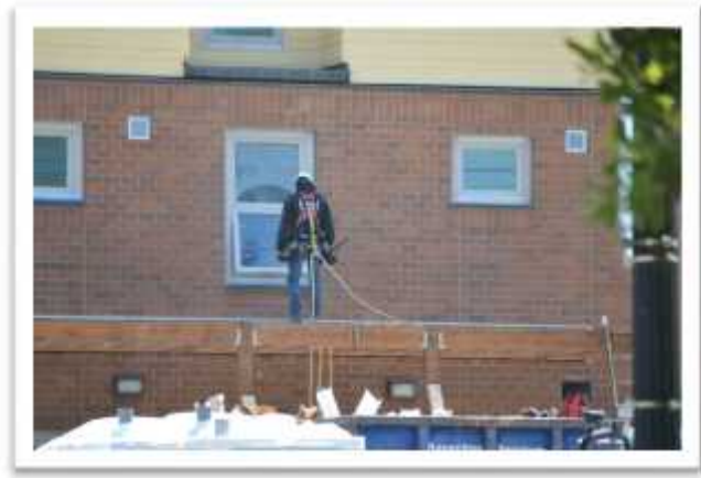
When working at heights, make sure you are using acceptable fall protection equipment, such as the harness in this photo.
