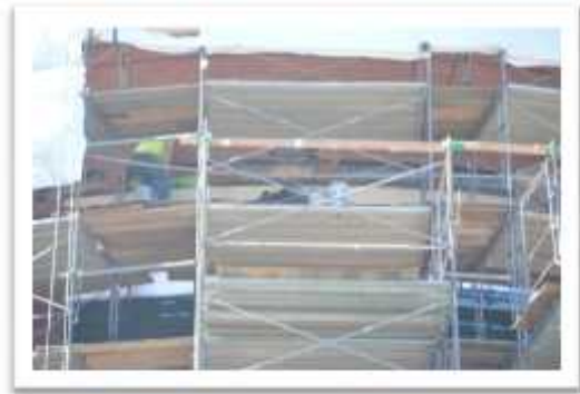
Scaffolding installation is an example of a task that should have a safe job procedure.
