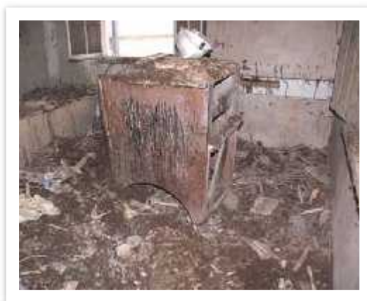
Pigeon droppings in an abandoned building
