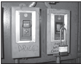
Main disconnect switch
